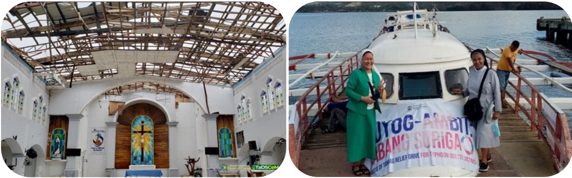
Left: Unroofed parish church of Sts. Peter and Paul; Right: Going home tired but happy - Sr. Odilia, OSB with Sr. Pem, LGC.
